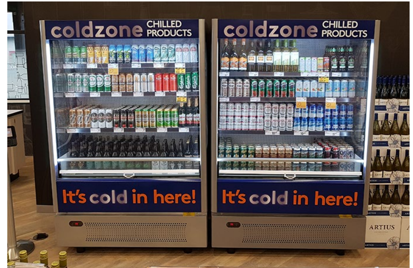
Open-front coolers at BCLS are equipped with a shade that is drawn at closing time every evening to reduce excessive cooling.
